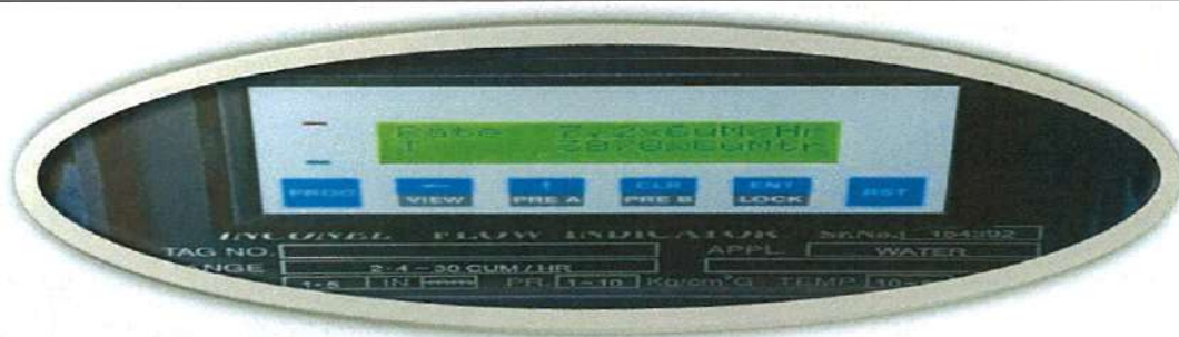
Digital Flow Meter Installed for water Consumption Monitoring at Crusher
