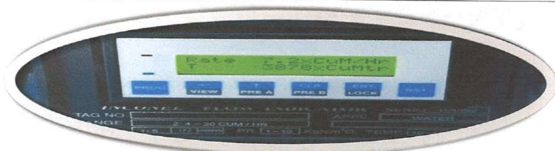
Digital Flow Meter Installed for water Consumption Monitoring at Crusher
